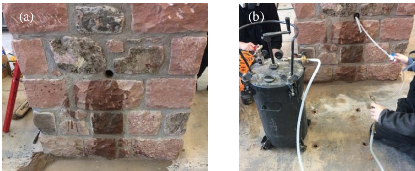
Fig. 4. Wall specimen preparation at ENU structural laboratory: (a) cleaning the hole in preparation of the anchoring system's installation; (b) injection of the cementitious grout in the fabric sleeve.
