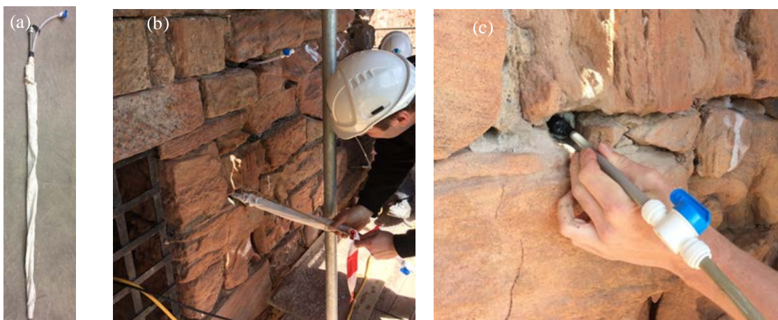
Fig. 2. (a) Cintec™ anchoring system; (b) installation of anchoring system and (c) injection of cementitious grout in the fabric sleeve, at the Latrine Tower, Bothwell castle.
